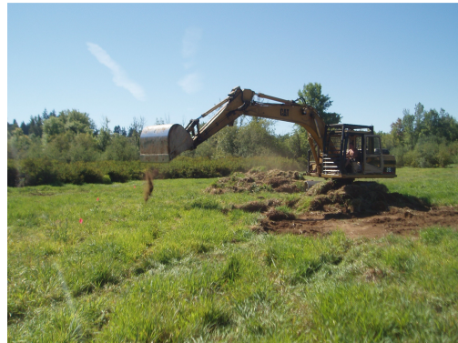
Excavator begins to remove sod of reed canarygrass and forming microtopographic swale at Shotwell's Landing.
